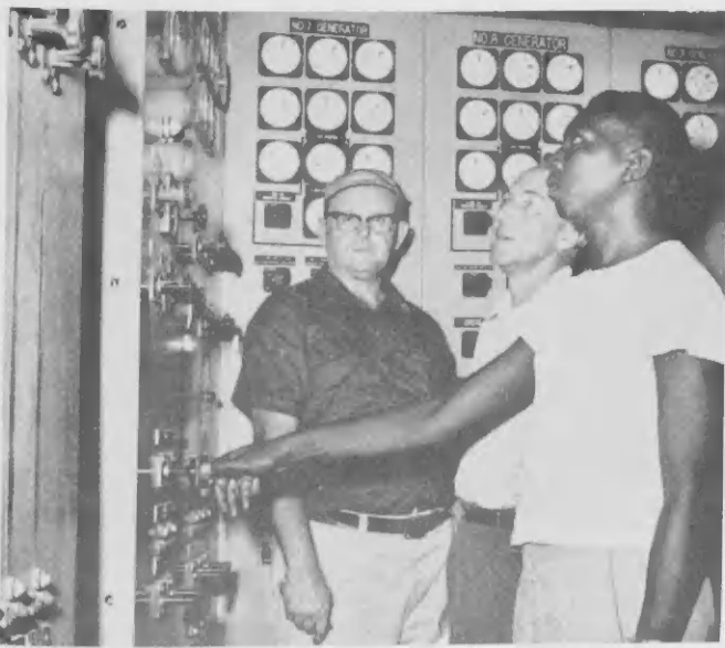
IN ONE of the moves preparatory to switching in the Balashi electrical source at Powerhouse No. 1, F. N. Clark turned on a synchroscope plug. Watching are W. R. Moore and C. R. Osborn, both of Utilities.
